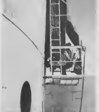
ELECTRIC WELDER builds up rows of shell plates, one requires eight hours to make one complete cycle around a tank.
